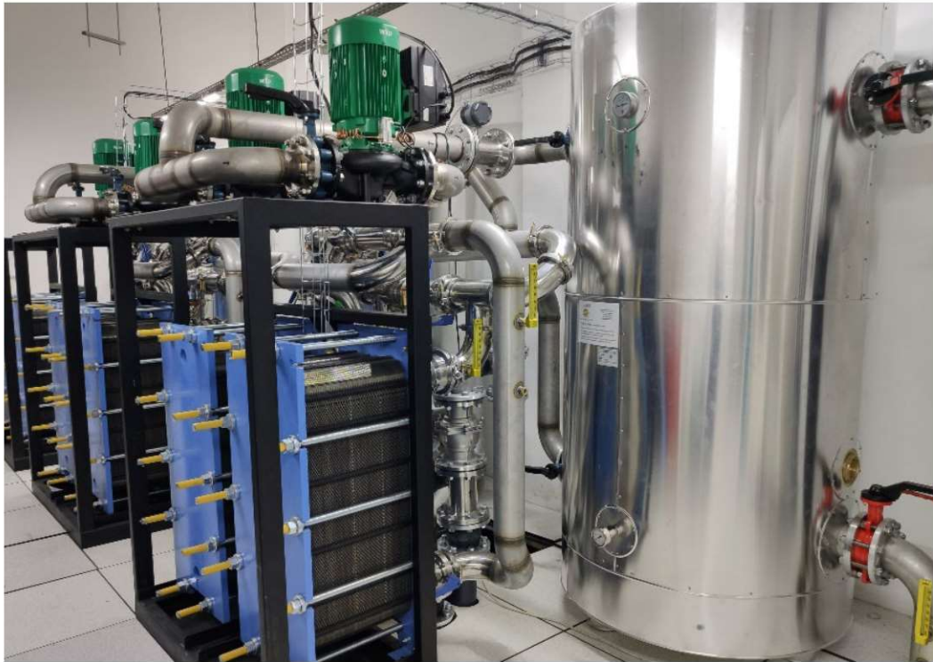
Pumps and Plate Heat Exchangers « behind the scene »
