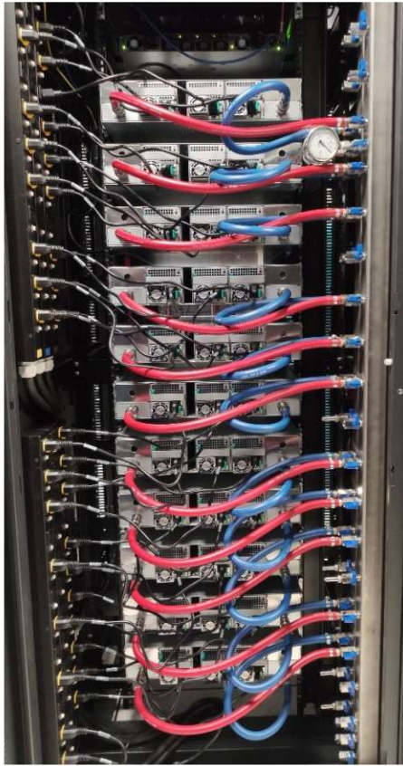
Rack rear view (with water hoses)
