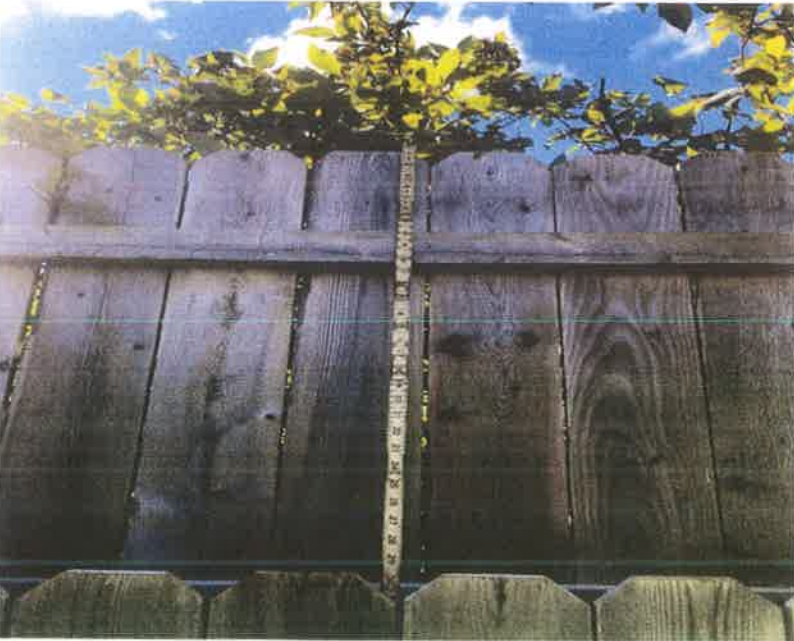
2.5 foot by 100 foot long well maintained vertical cedar extension placed 2017. Supporting side is 41 inches, nailed to stringers.
